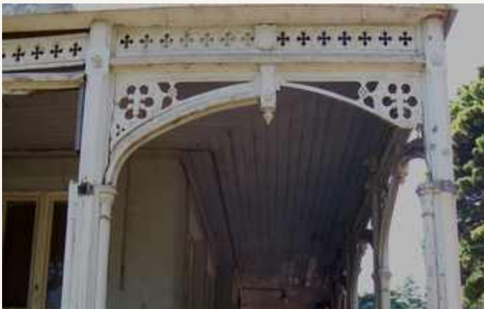
BEFORE — THE ORIGINAL VERANDAH, DECAYED
